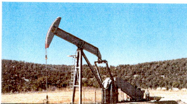
Figure 2: Walking Beam Pump for CBM Water Extraction
