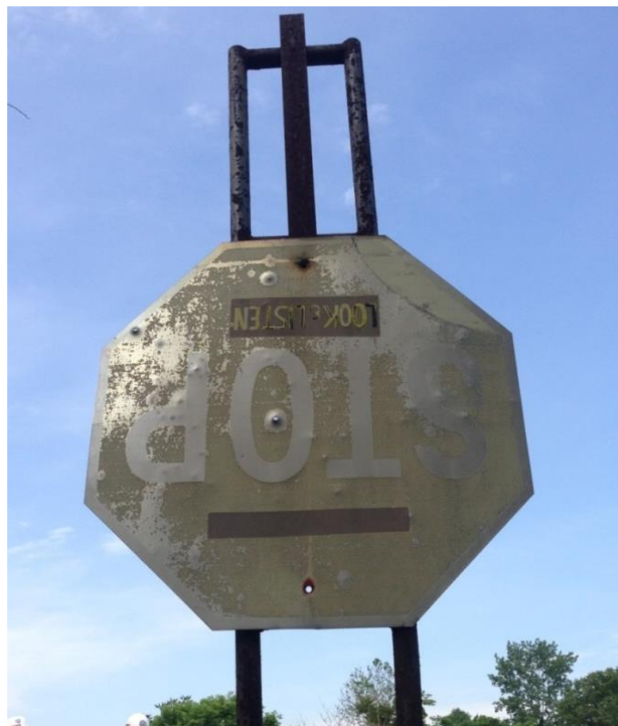
Figure 9. Detail view of STOP sign at grade crossing.
