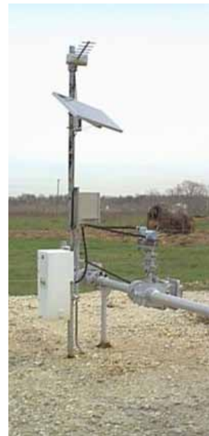
Instrument box with solar panel and antenna
