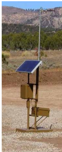
Valve with solar power and telemetry
