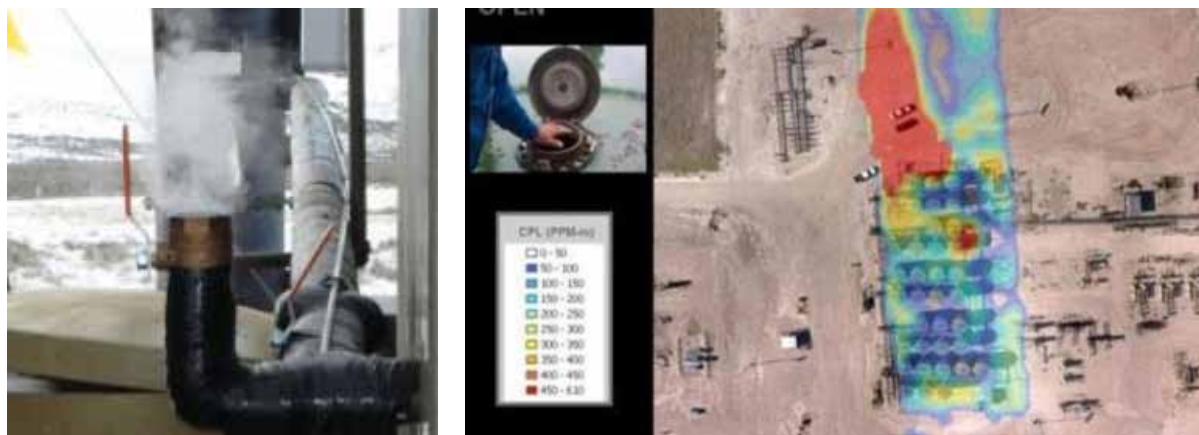
Leaking ball valve
