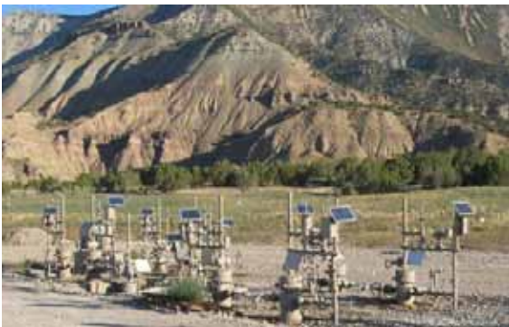
There are sixteen wells on this well pad.
