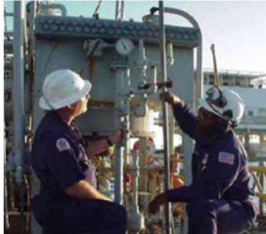
Looking at controller
