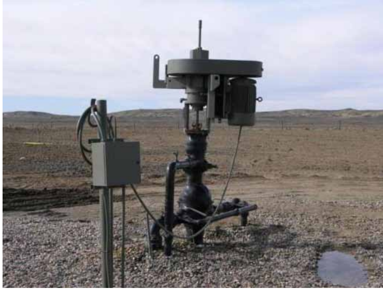
Electric wellhead pump
